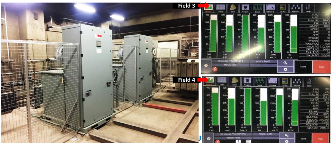
Installed HFTR in 3 rd and 4 th Field of ESP
